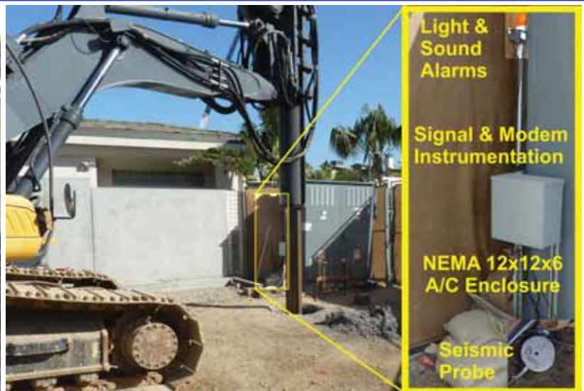
Typical AC Modem On-site Seismic Installation
