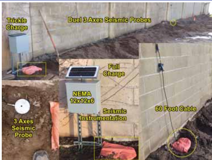
Typical Dual DC On-site Seismic Installation
